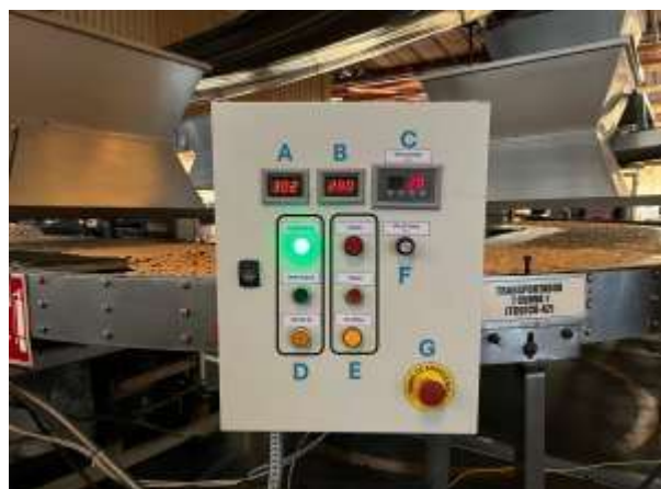
Figure 6. Control panel in full operation. A), B) Temperature monitors, C) Speed, D), E) Start, stop, and alarm reset, F) Belt speed control, G) Emergency stop. Source: Authors.
